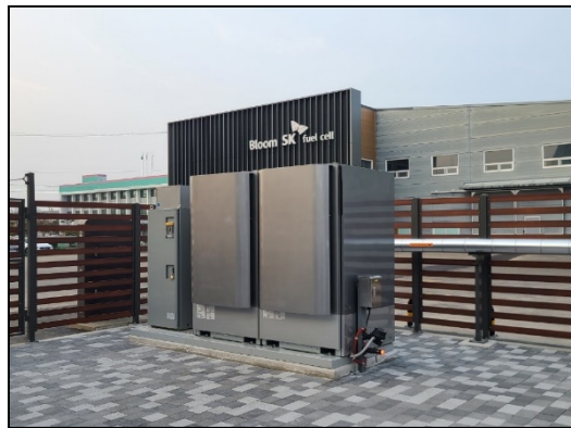
[SOEC Demonstration Facility]
